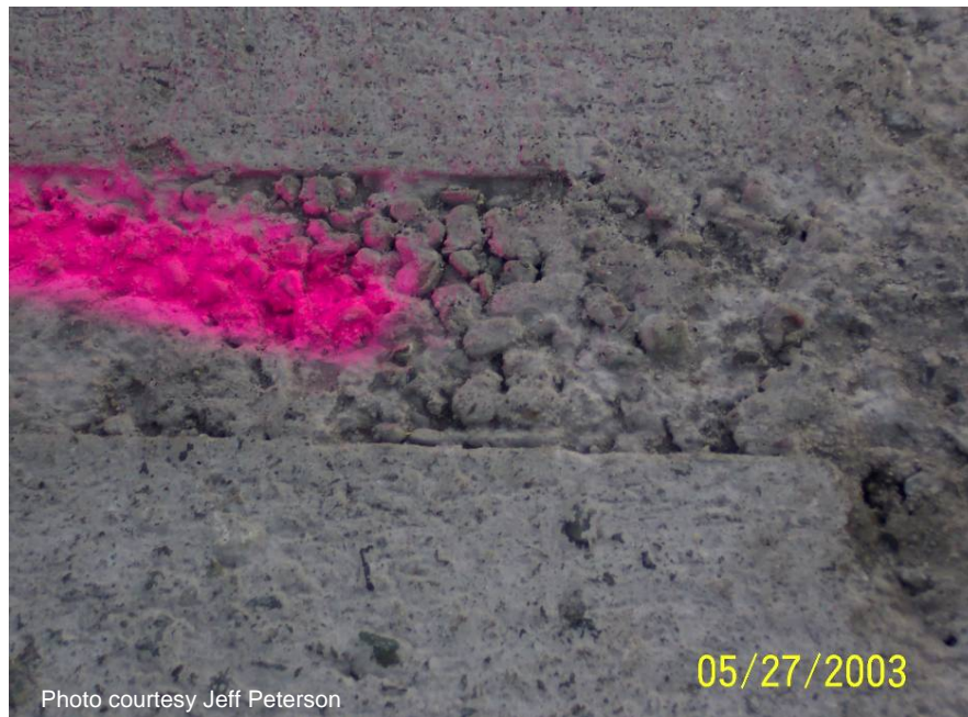
Figure 46 Insufficient consolidation of patching material.
