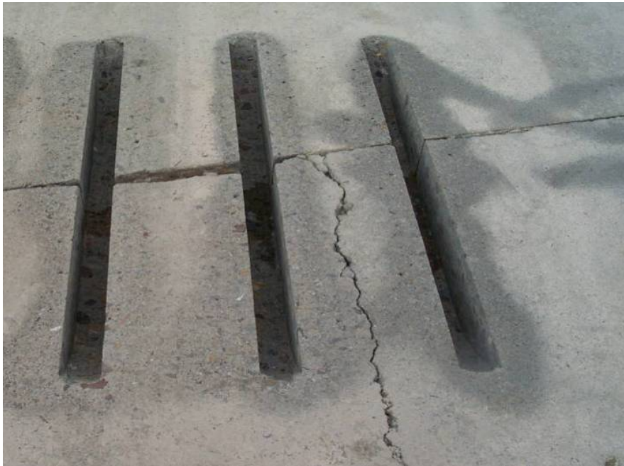
Figure 17 Dowel bar slots aligned to miss an existing longitudinal crack.
