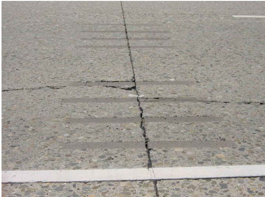
Figure 19 Failure of dowel bar slot placed over existing longitudinal crack.
