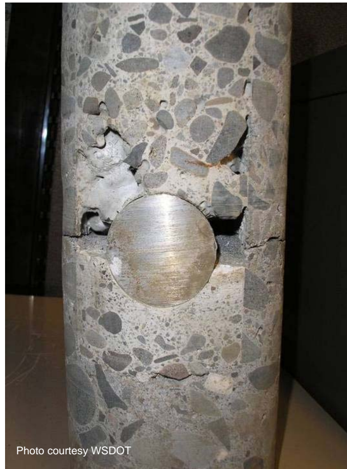
Figure 69 Poor consolidation around bar.
