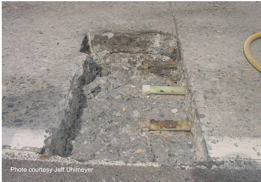
Figure 58 Corroded epoxy coated dowel bars.
