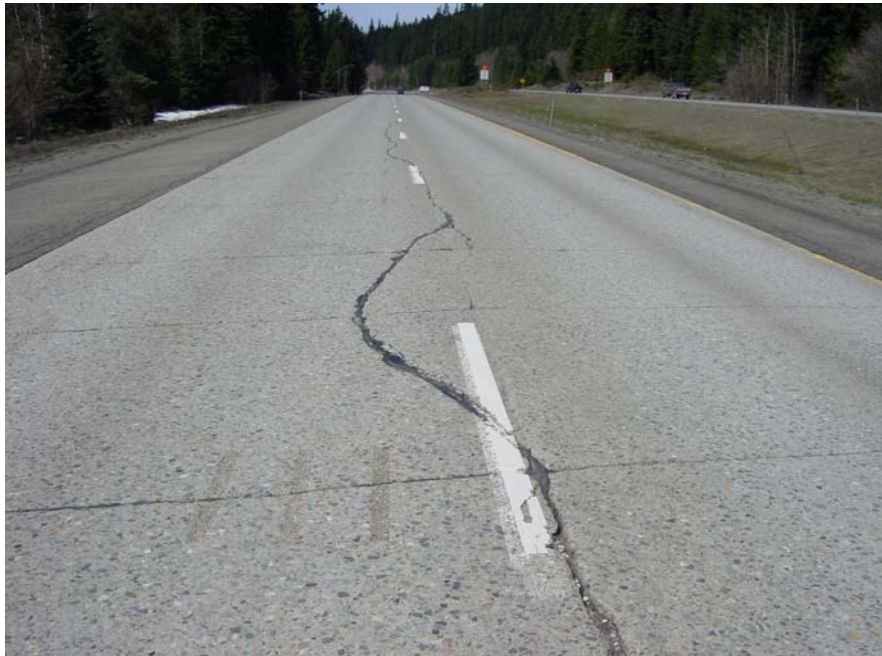
Figure 18 Left wheelpath dowel bar slots not installed to avoid existing longitudinal crack.
