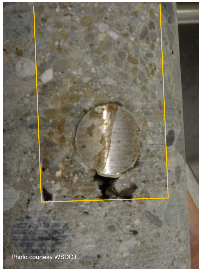
Figure 68 Poor consolidation beneath bar.
