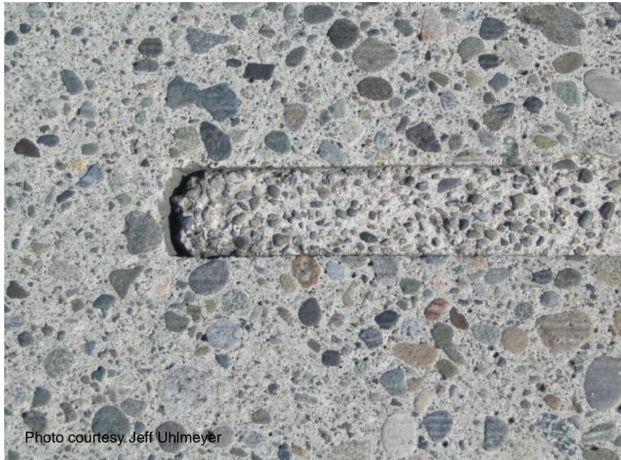
Figure 43 Patching material bond failure.
