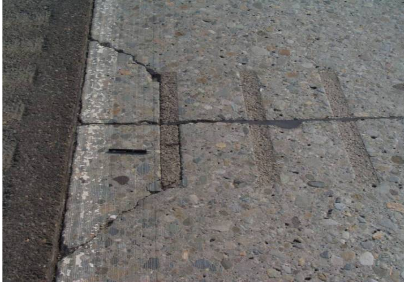
Figure 15 Distress due to dowel bar slot cut and/or chipped too deep.
