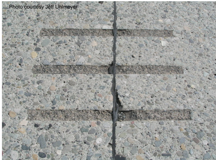
Figure 45 Spalling of patching material.
