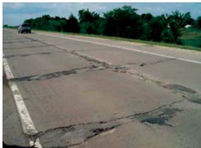
Figure 5-5. Concrete pavement with severe joint spalling (photo courtesy of Todd LaTorella, MO/KS ACPA)
