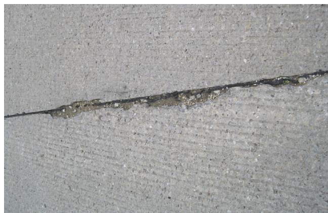
Figure 1-4. Joint deterioration (Photo courtesy of Jim Grove, FHWA)
