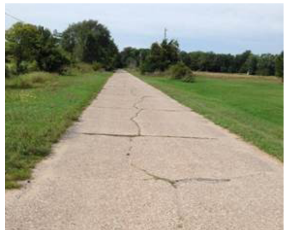
Figure 1-2. Moscow street in 2014 (photo courtesy of Kurt Smith, Applied Pavement Technology, Inc.)
