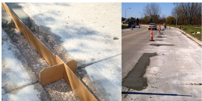
Figure 5-2. Milled joint for removal of spalling (left photo) and finished PDR (right photo, courtesy of City of West Des Moines, Iowa)
