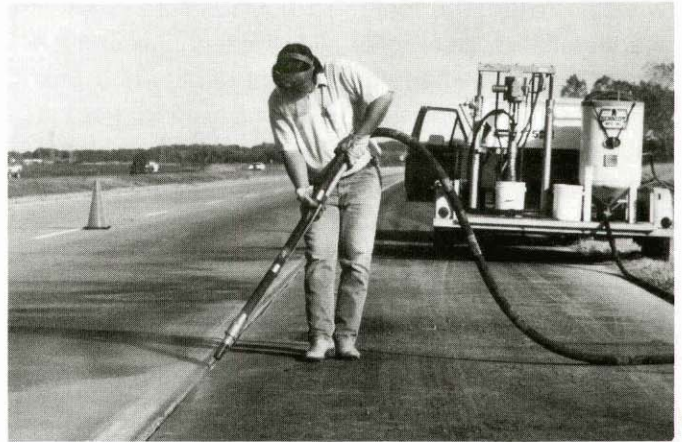
Figure 14 Sandblasting a shoulder joint. Note the angle and close proximity of nozzle to the reservoir.
