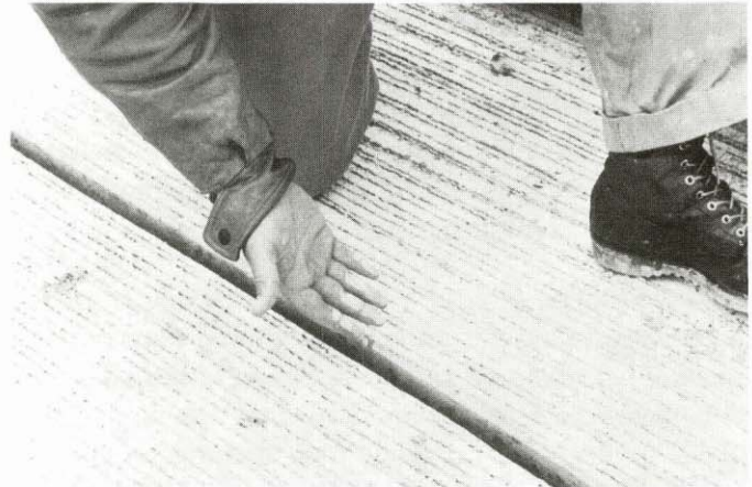
Figure 16 Noticeable dust on inspector’s fingers.
