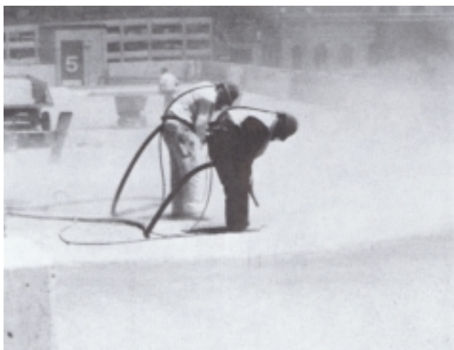
Fig. 1. Sandblasting can clean any size or shape surface—horizontal, vertical, or overhead and remove weak, deteriorated concrete.
