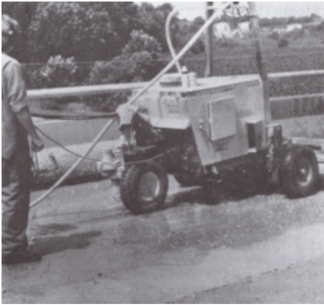
Fig. 6. Waterblasting can be used to clean a surface lightly without abrading the concrete or it can abrade the surface and remove weak concrete. The equipment shown removes the concrete surface (for a future overlay) with fine jets of water at pressures between 6000 and 17,000 psi (41 and 117 MPa). Wand-type waterblasting equipment is also available.
